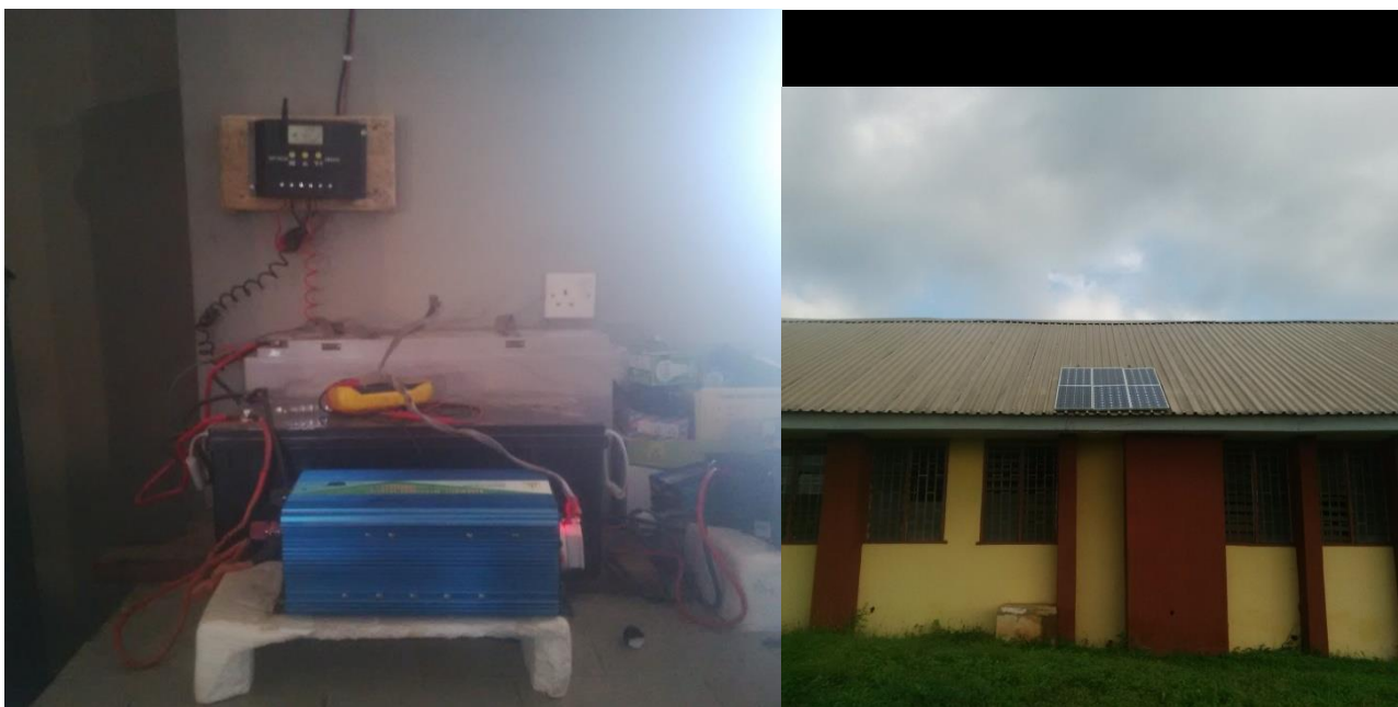
Plate 1: The view of the installed 40 W digital charge controller, 400 AH solar battery and six 80 W (480W) mono-crystalline photovoltaic solar panels.
